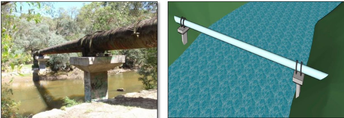
Figures 18 and 19 above illustrate indicative pipe bridge and supports across a stream
