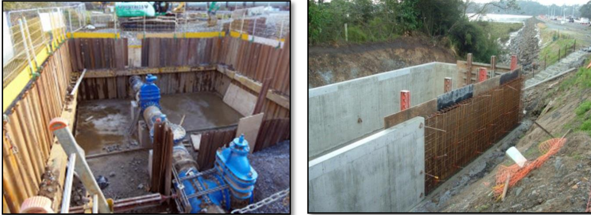
Figures 15 and 16 above show examples of valve chambers using sheet pile (left image) and tilt slab concrete (right image)
